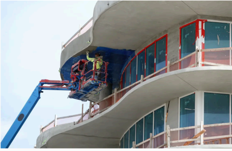
Work continues on the Pier Sixty-Six project in Fort Lauderdale on Thursday. The project design reflects the aesthetics of the original building. (Lise Cavaretta/South Florida Sun Sentinel)
