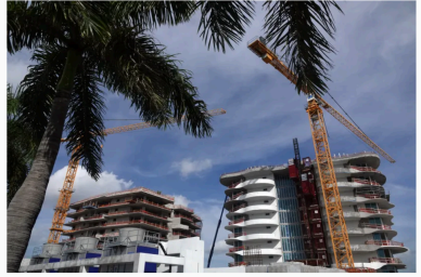
Work continues on the Pier Sixty-Six project in Fort Lauderdale on Thursday. The project design reflects the aesthetics of the original building. (Lise Cavaretta/South Florida Sun Sentinel)
