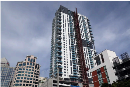
Work on the Related tower rental project on Federal Highway in Fort Lauderdale. (Lise Cavaretta/South Florida Sun Sentinel)
