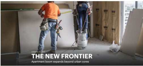
Construction workers work on the 102-unit Town Square apartments in Pompano Beach, which will be completed in November of 2023. SOURCE: SOUTH FLORIDA BUSINESS JOURNAL
