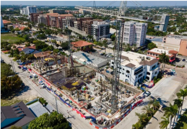
Aerial photo of construction of Royal Palm Residences, a luxury condominium being built in Boca Raton. Group P6
