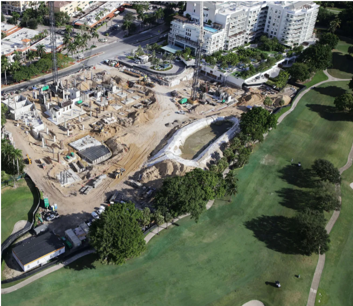
Aerial view of construction taking place on the second phase of Alina Residences, a luxury condominium complex in Boca Raton. Durée & Company, Inc.
